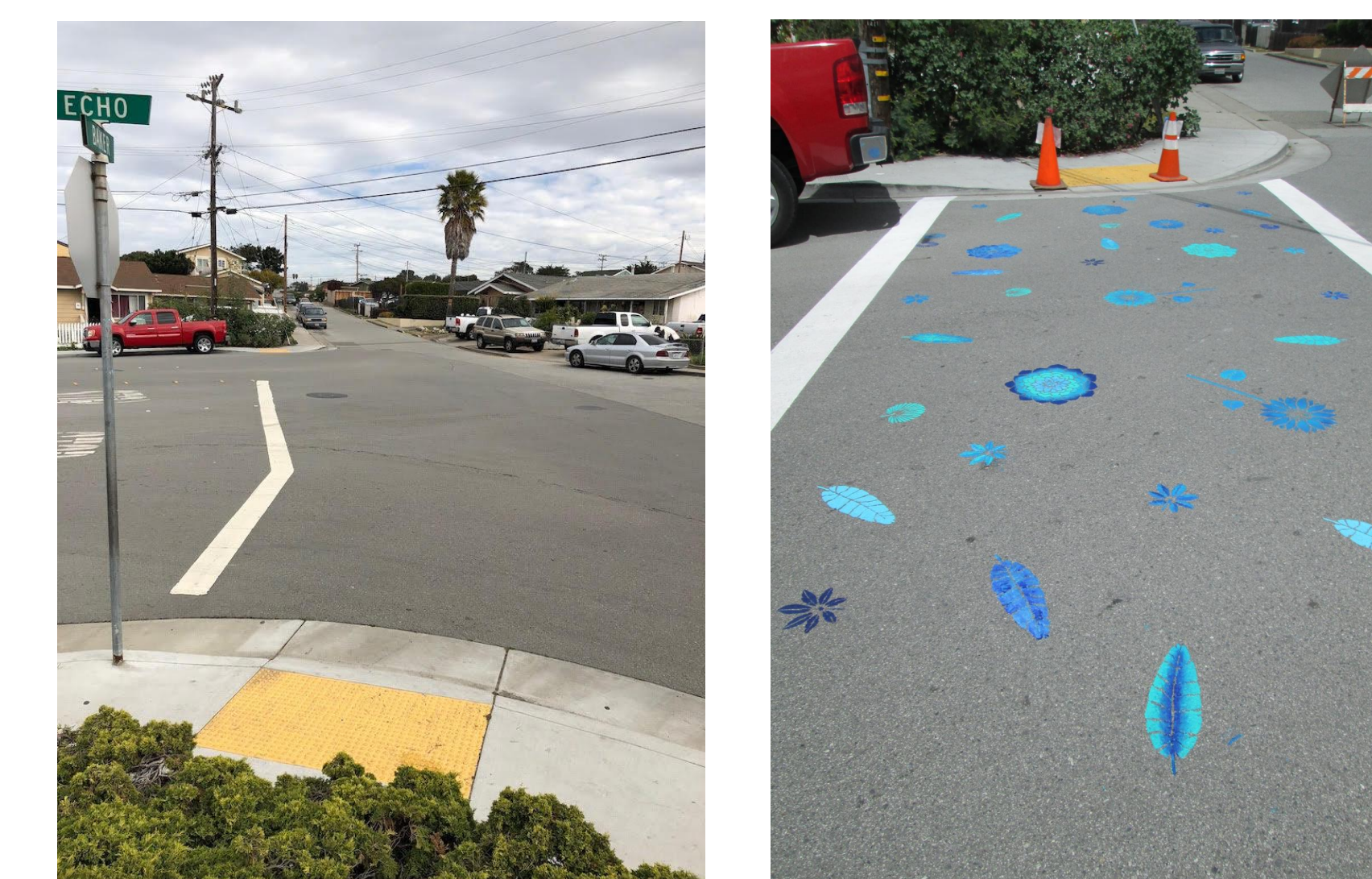
Before (left) and after (right) the crosswalk installation on Echo Avenue. STU added colorful flowers and leaves between the white lines painted by the City of Seaside
